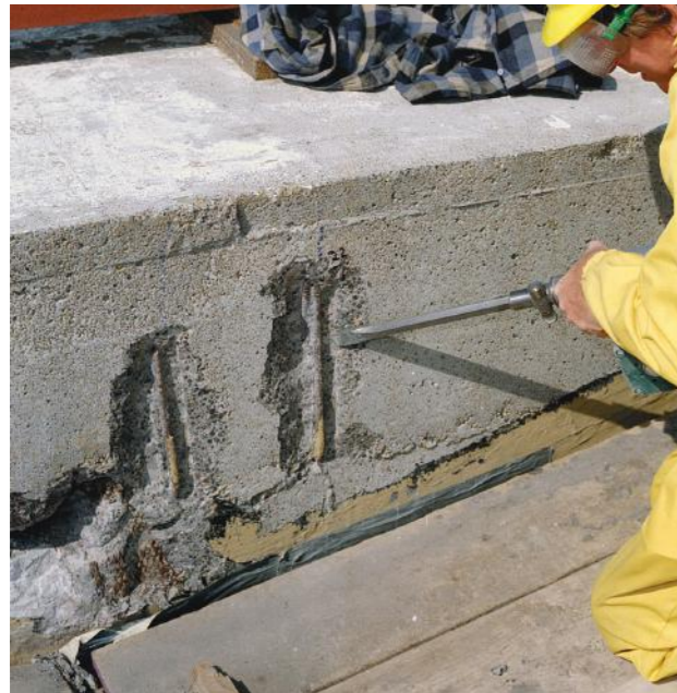
Damaged concrete structure
