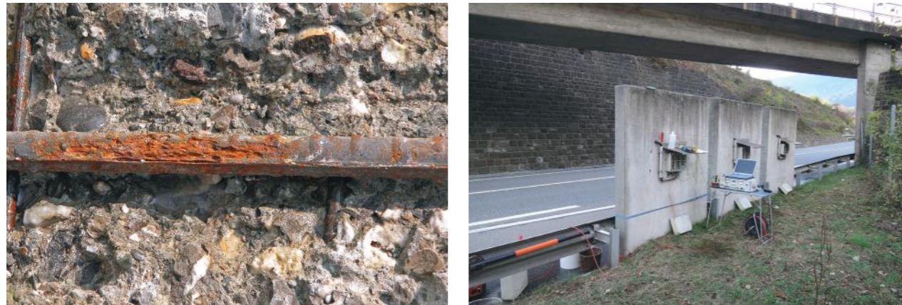
Damage to concrete structure due to insufficient concrete cover and low concrete quality.
