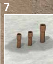
Leaking Penetrations i.e. Pipe Penetrations
