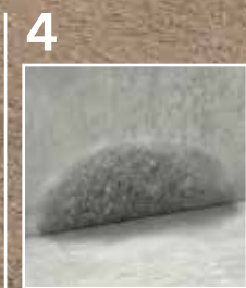
Leaking Areas of Voids i.e. Honeycombing
