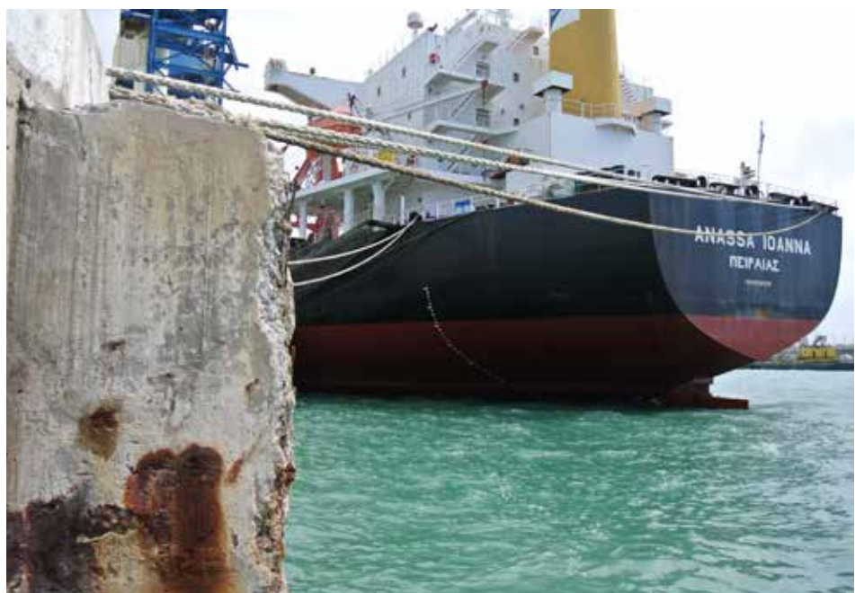
Reinforcing steel corrosion in a pier.
