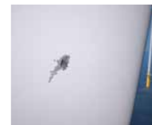
Structural composite damage.
