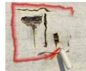
Identify and assess damage.
